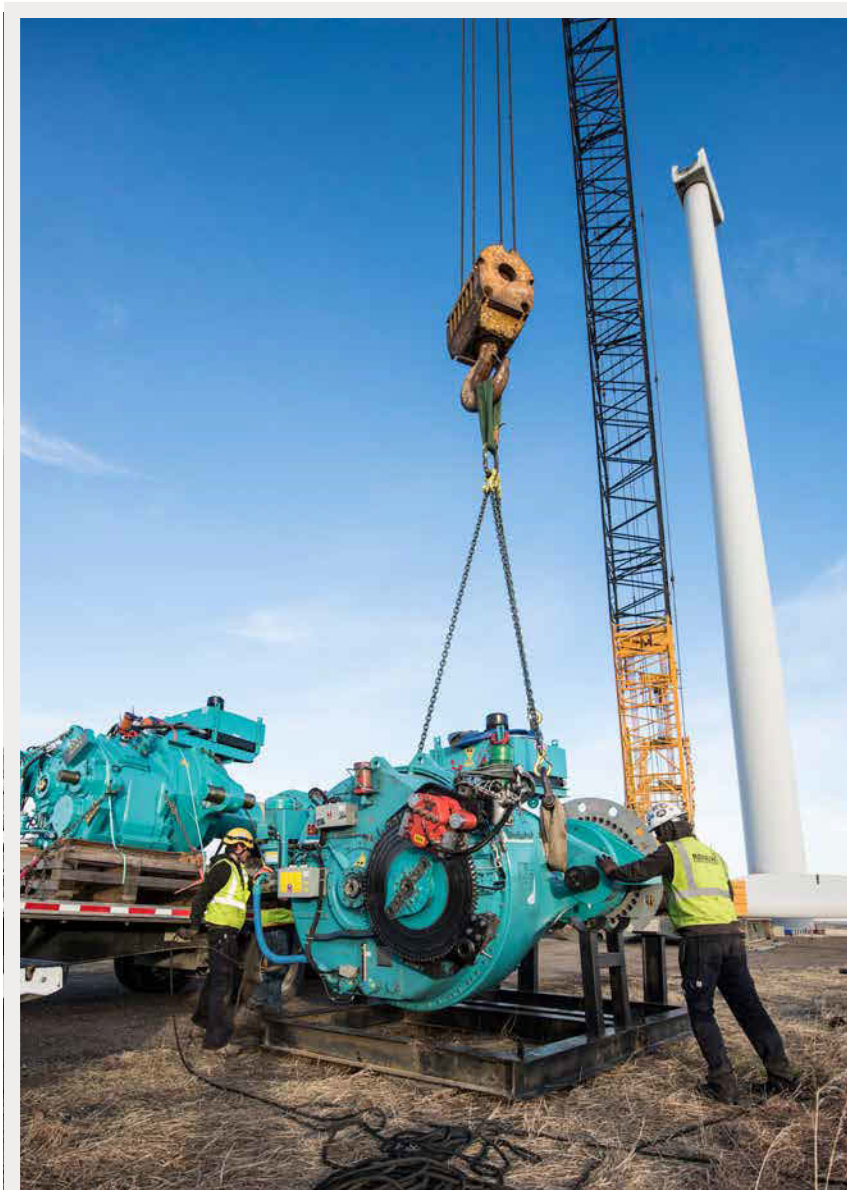
Making the change. Wind power plant operation and maintenance costs account for as much as 20% to 50% of the wind power purchase agreement price and generally increase as wind power plants age. Photo by Dennis Schroeder, NREL 49409
