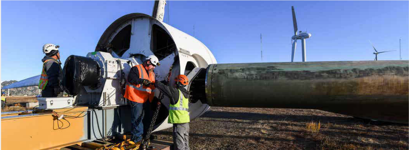
NREL engineers and technicians installed the Segmented Ultralight Morphing Rotor demonstration rotor onto the two-bladed Controls Advanced Research Turbine at the NWTC on October 5, 2018. Photo by Dennis Schroeder, NREL 53473
