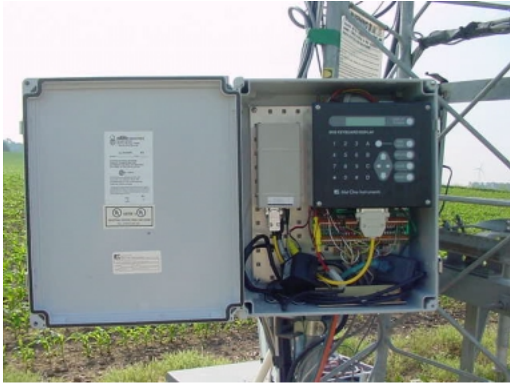
Figure 12. Met One logger installed at tower 101
