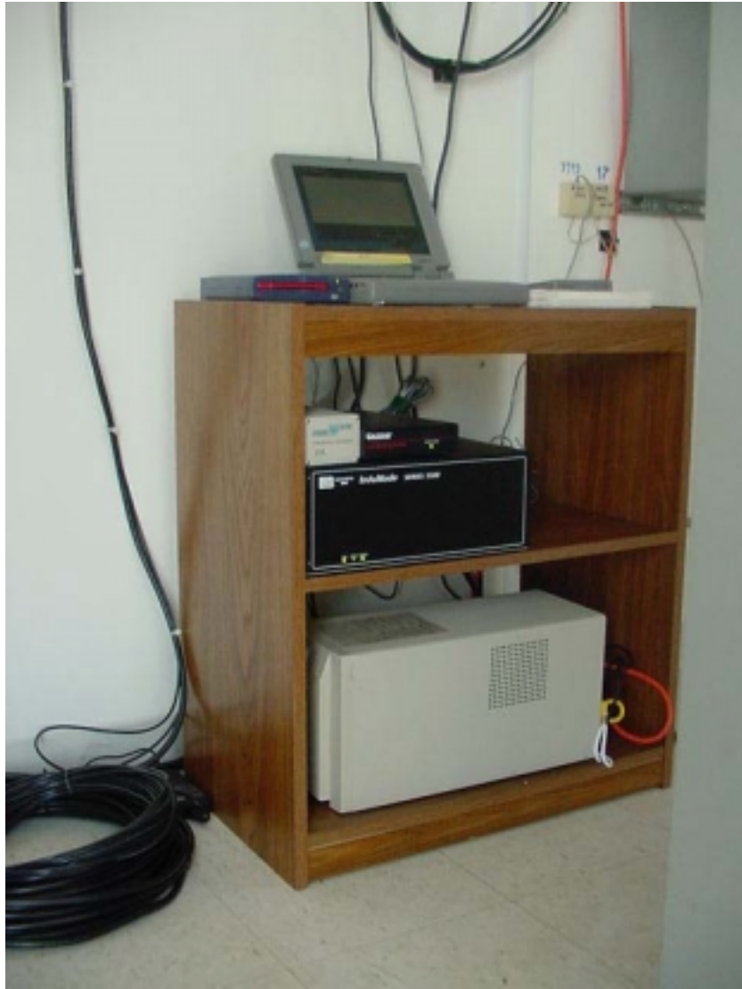
Figure 17. InfoNode installation at Golf interconnect building
