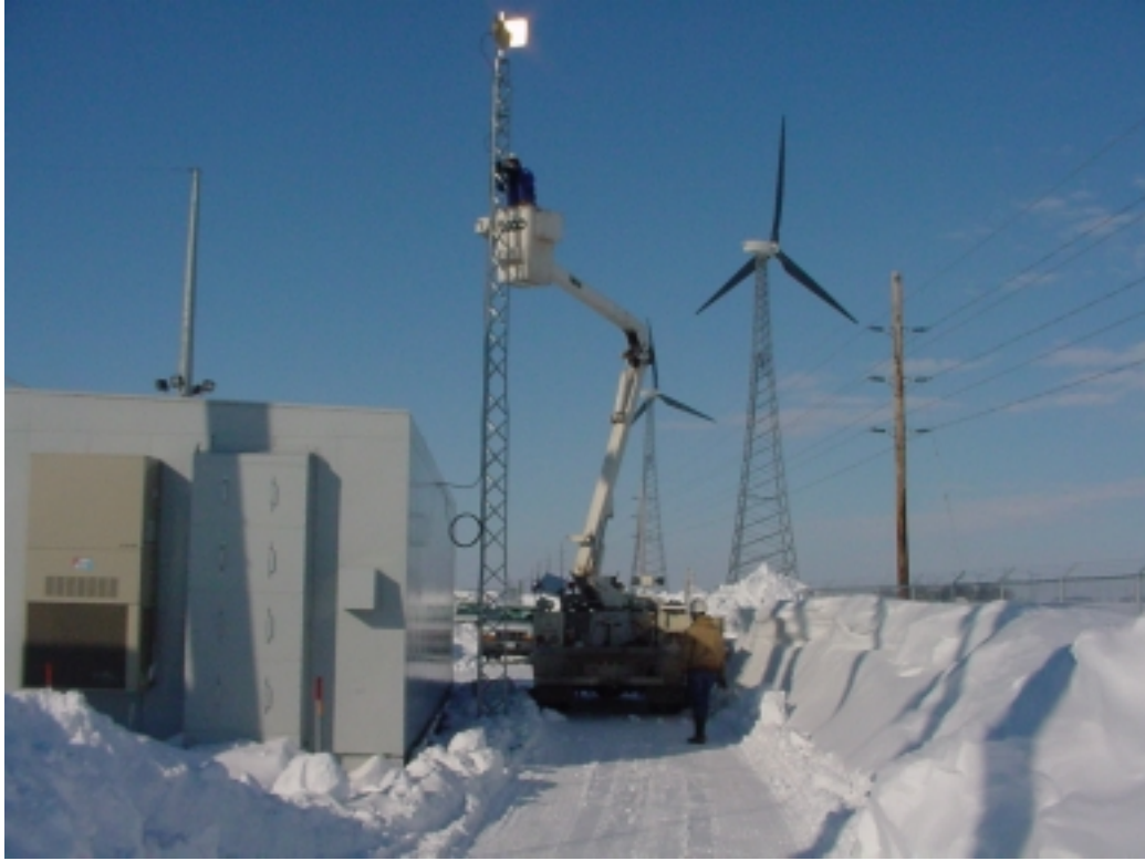
Figure 11. Substation antenna for collecting met data
