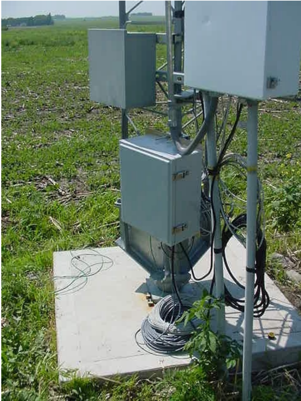
Figure 19. Met One logger installed at tower 6
