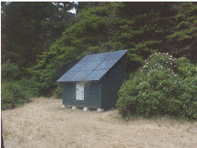
Figure 1. Photo of 1080 W PV array atop structure housing fuel cell, batteries, inverter and controls.
