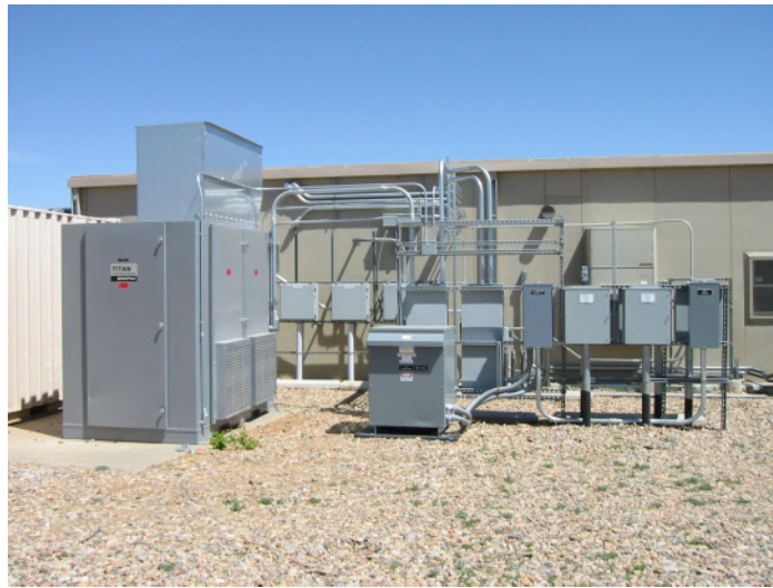
Figure 29. A 165-kW Titan load bank (on left)
