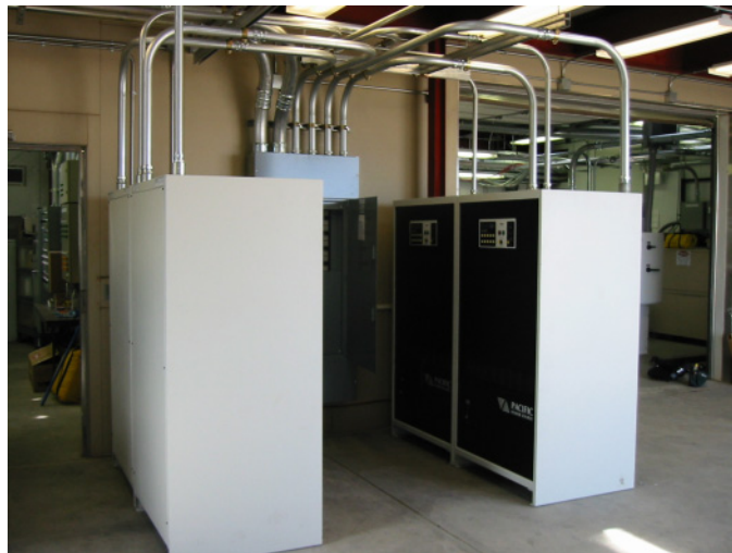
Figure 28. 200-kW grid simulator array
