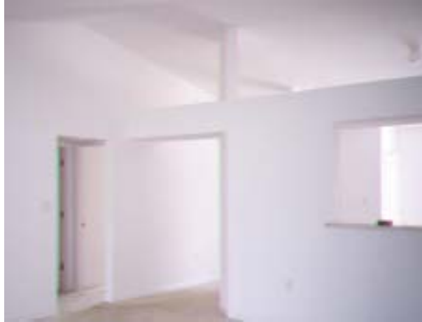
Figure II-12. Photo of boxed-in ductwork main crossing main living area, running from air handler to bedrooms
