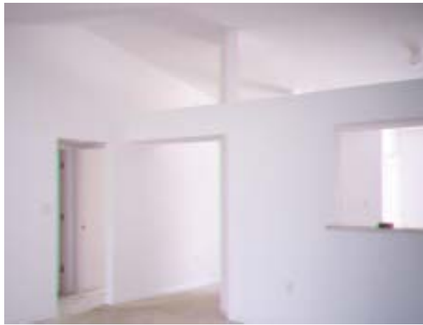
Figure II-6. Boxed-in main duct between kitchen and living room
