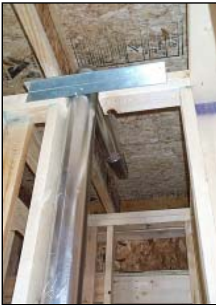
Figure I-32. Supply duct in wall cavity up to second floor
