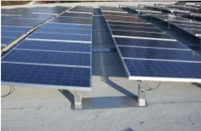
Figure 8. View of baseplate with both RoofJacks supporting PV module assemblies.
