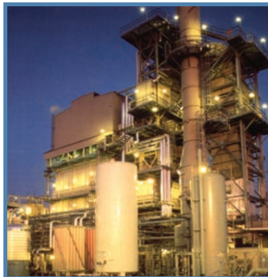
Figure 3.1.1 Centralized Hydrogen Production Facility
