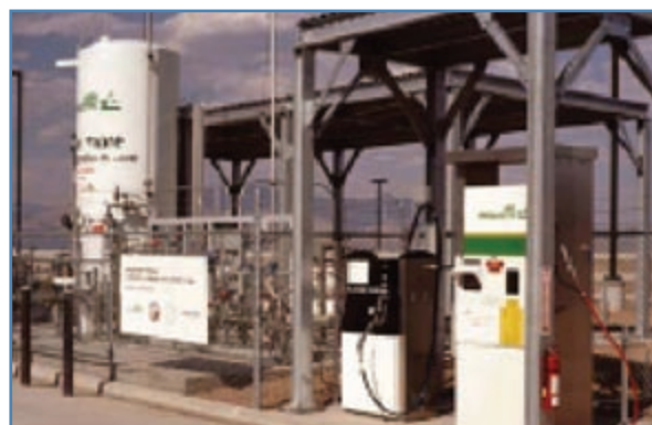
Figure 3.7.1 Air Products Hydrogen Fueling Station in Las Vegas, Nevada
