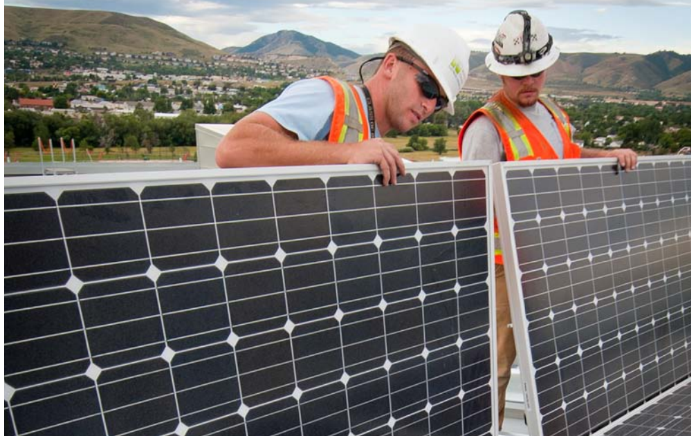
A PPA funded 1.6 MW of photovoltaics installed on the Research Support Facility at the National Renewable Energy Laboratory. Photo by Dennis Schroeder, NREL/PIX 18482
