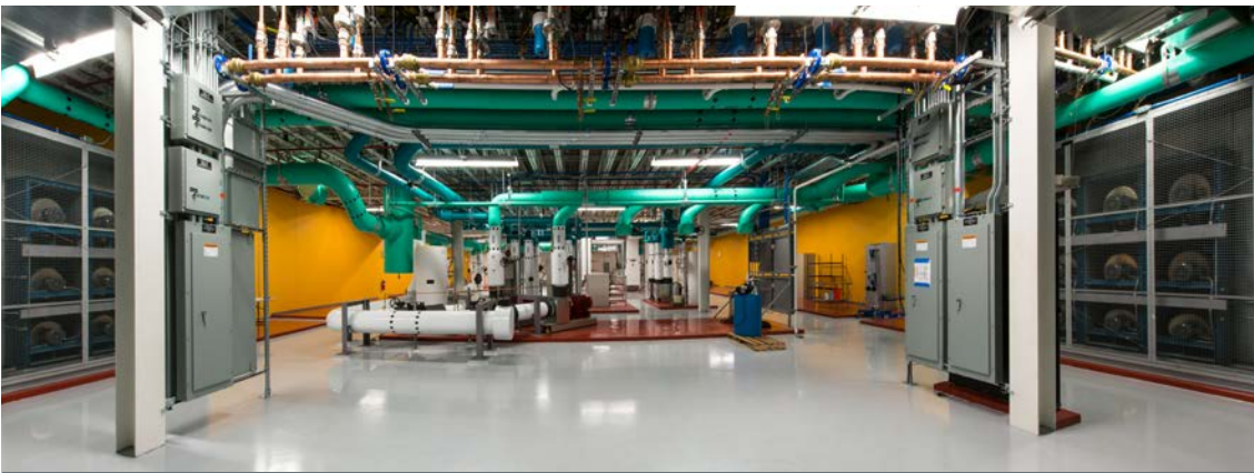
Pumps provide cool water to the server racks in the ESIF HPC data center. Traditional direct expansion cooling is not used.
