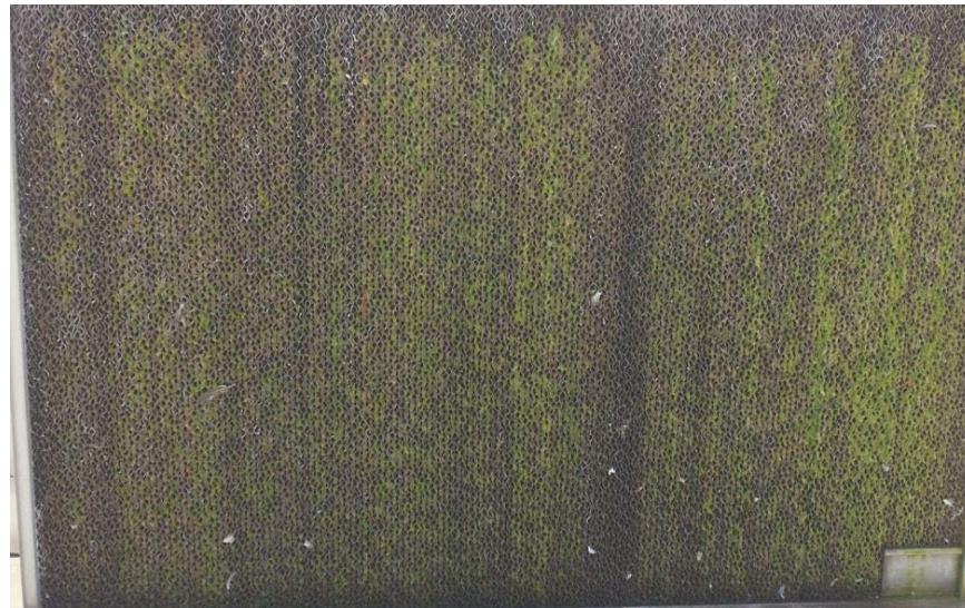
Figure 35. Direct evaporative media with algae buildup
