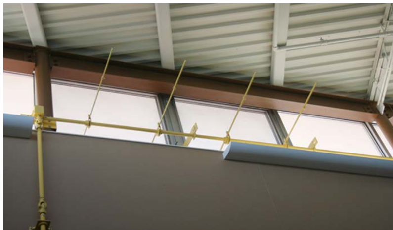
Figure 8. Operable clerestory windows at the Lussier Community Education Center in Madison, Wisconsin
