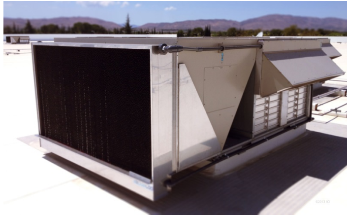
Figure 32. RTU with DualCool hybrid system installed, which includes evaporative precooling and evaporative condensing
