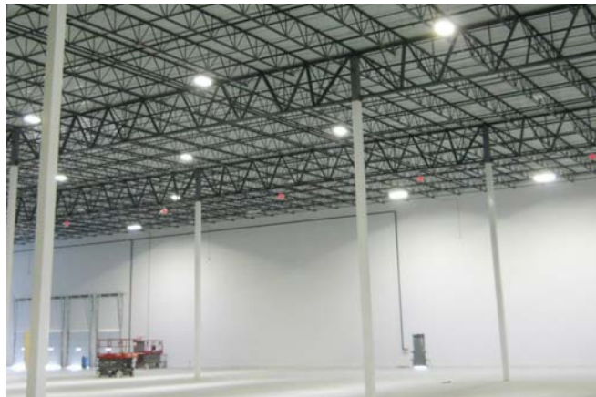
Figure 20. High bay LED in a warehouse
