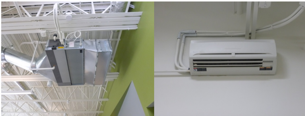
Figure 23. Two types of VRF indoor units
