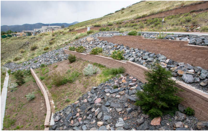
A multiyear effort to stabilize the hillside west of the Field Test Laboratory Building was deemed successful in 2021. Photo by Werner Slocum, NREL 68353
