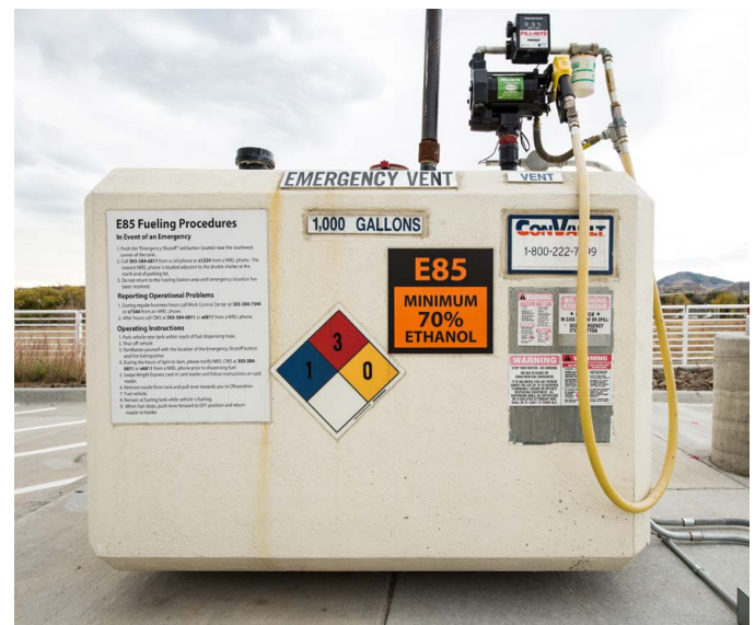
A 1,000-gallon (4,546-L) aboveground storage tank on the STM Campus containing gasoline is maintained to refuel site support vehicles. Photo by Dennis Schroeder, NREL 32151
