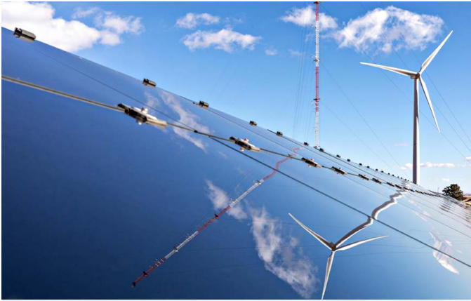
A wind turbine is reflected in a photovoltaic array at the Flatirons Campus. Photo by Werner Slocum, NREL 66364
