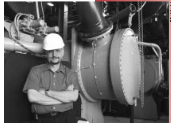
Project Coordinator Steve Krstulovich with Fermilab's new 1400-ton, high-efficiency chiller.
