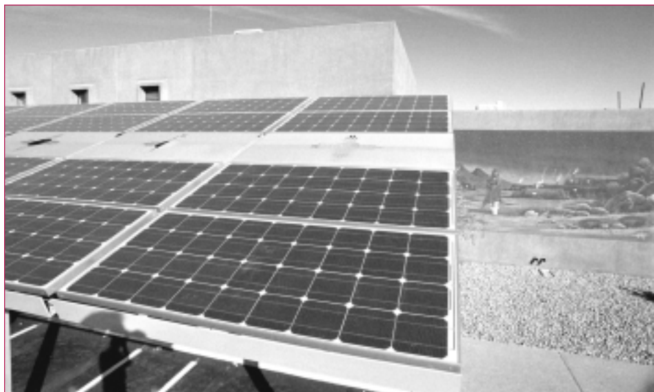
At the Indian Pueblo Cultural Center in Albuquerque, NM, this PV carport stands ready to impress more than 400,000 visitors each year. The system delivers about 23 megawatt hours of clean electricity annually to the local utility grid, making it the largest commercial PV system in New Mexico. NCPV engineers from Sandia were responsible for the project's electrical design review.
