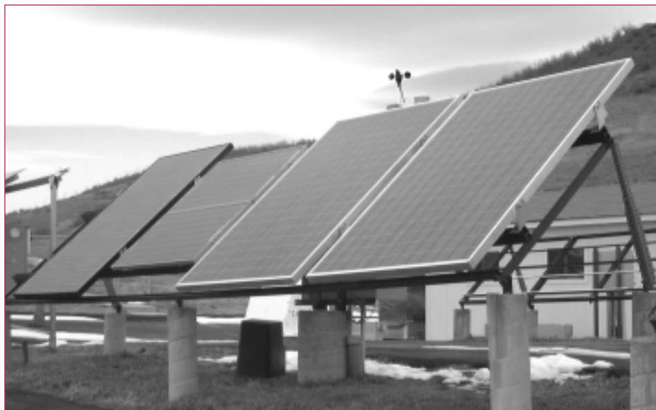
AC PV modules that have a DC/AC inverter attached directly to the back side are being monitored for long-term performance and reliability by the PV Program on this new, specially designed testbed at NREL's Outdoor Test Facility. The four modules pictured are (from right to left) BP Solarex/Advanced Energy Systems 240 W, Evergreen Solar 90 W, and Ascension Technology 275 and 250 W.
