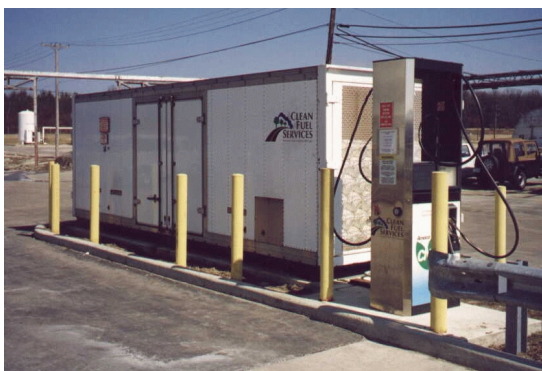
Figure 1. On-Site CNG Fueling Facility
