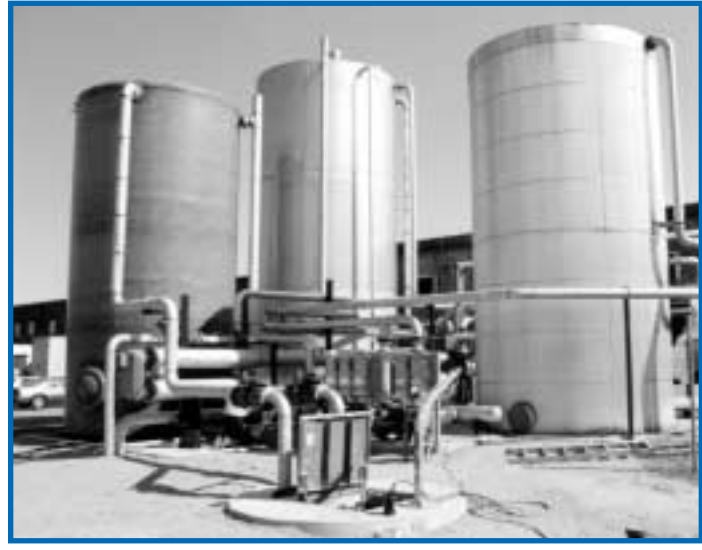
Wastewater storage tank (left in photo), warm water storage tank (center), original hot water storage tank (right), with equipment and wastewater sump in foreground.
