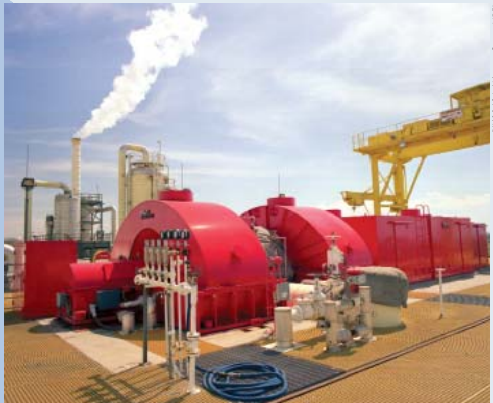
This geothermal power plant in the Imperial Valley in southeastern California generates electricity from steam produced underground in the Salton Sea geothermal reservoir. DOE was a partner in this project.
