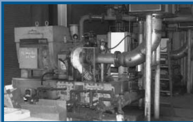
U. S. Steel replaced old, unreliable rotary screw compressors with 600-hp centrifugal compressors, shown here, at its Edgar Thomson Plant in Braddock, Pennsylvania.
