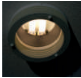
Energy-efficient lights cut down on the building's energy costs.
