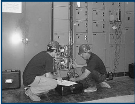
A data logger is set up to capture real-time motor systems data.
