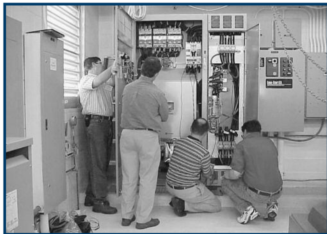
Workshop participants gain hands-on experience with PSAT by conducting tests and collecting measurements at a VPI Water Authority pumping facility.
