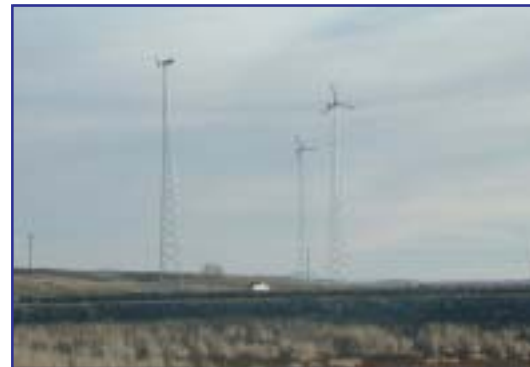
Three Bergey wind turbines are on the north side of the Browning Waste Water Treatment Plant aeration ponds.
