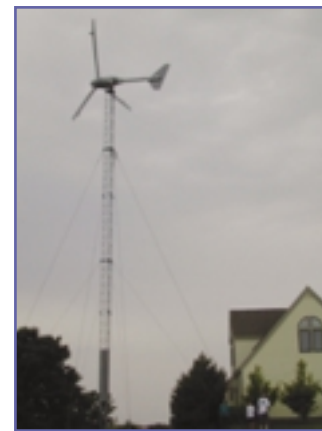
Figure 18. A guy wire failed on the Evans Residence Bergey Excel-S/E 10 kW.
