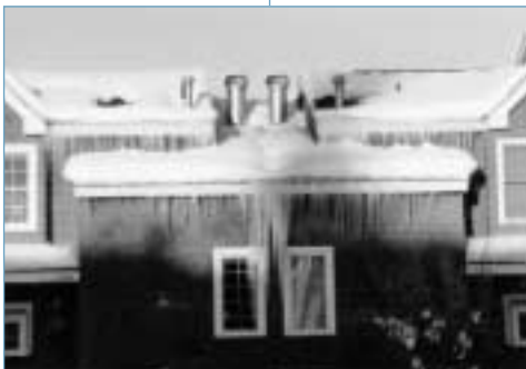
Before weatherization, warm air leaks caused ice dams, hazardous icicles, and structural damage in this low-income home.
