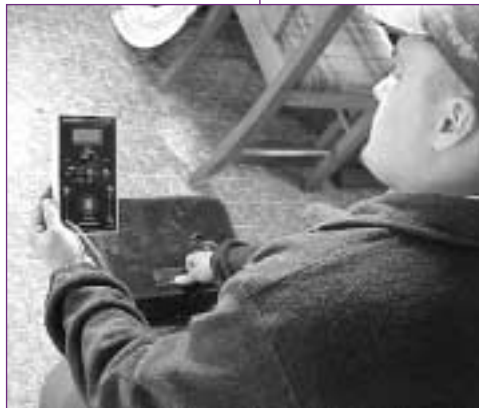
Delaware crews use a digital manometer, like this one, to identify air pressure imbalances.
