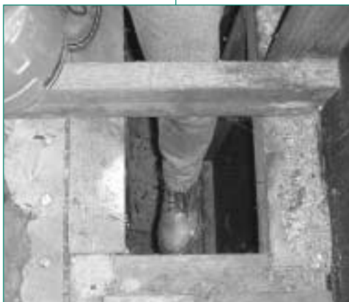
A weatherization technician illustrates a common point of air infiltration, an open chimney bypass. The crew will seal the bypass and insulate the area to reduce heat loss.
