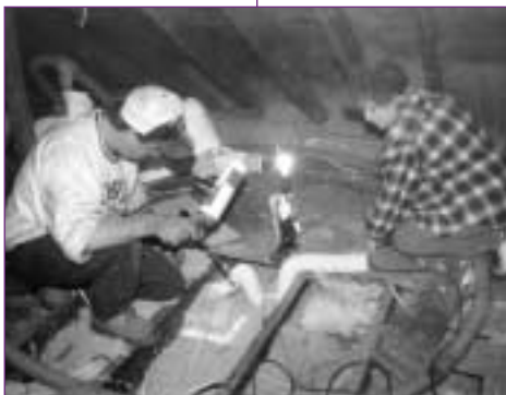
Weatherization crew installs insulation in the attic of a New Jersey home.
