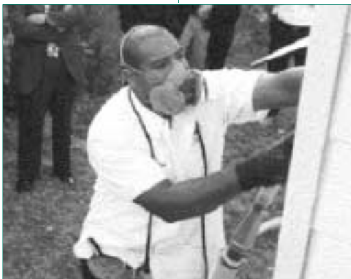
During a public demonstration, an Ohio weatherization worker installs sidewall insulation to increase the energy efficiency of the home.
