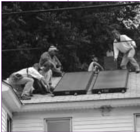
Weatherization crew installs a solar hot water system in a low-income Pennsylvania home.
