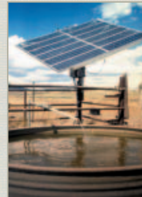
Ute Mountain Indian Reservation PV Water Pumping
