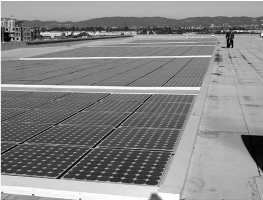
The rooftop solar system at the USPS Marina del Rey Center in Los Angeles is based on a technology that uses polystyrene foam backing behind the PV cells, which also provides more thermal insulation to the building; the system should save about $25,000 per year in energy costs.
