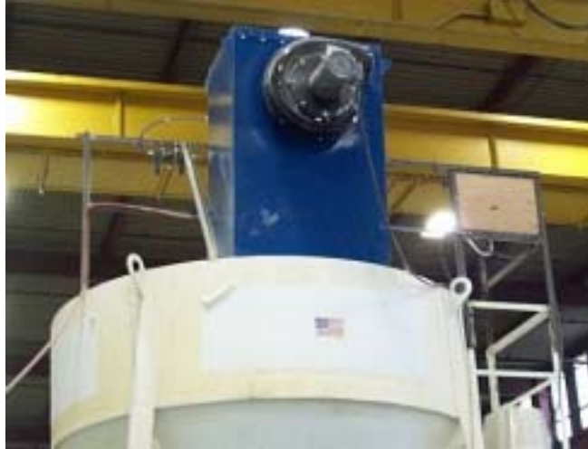
Figure 13: Dust Containment Box on Dry Goods Silo
