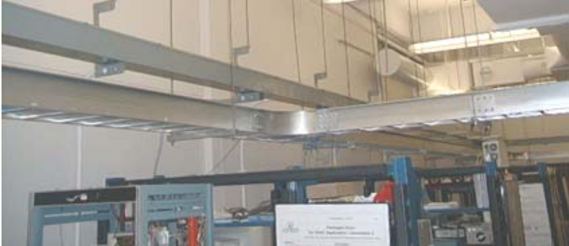
Figure 156: Photograph of cable tray system that forms the backbone of the laboratory-scale microgrid
