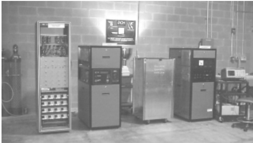
Figure 2-1. The testing area and test equipment (From left: hydrogen tanks, switch-mode load bank, fuel cell cabinet, incandescent load bank, and electronics cabinet)
