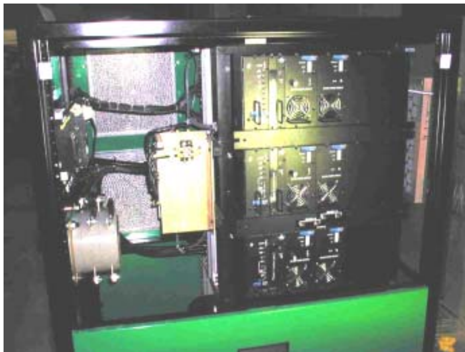
Figure 2-6. Right side of the electronics cabinet (Shows the power electronics, boost converters, and inverters)
