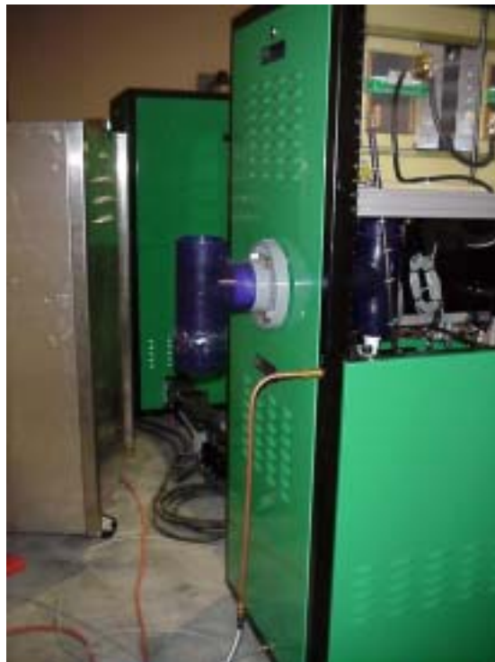
Figure 2-4. The back of the fuel cell cabinet (The large blue tube is the exhaust tube in which warm, humidified air is allowed to vent to the atmosphere; the small copper tube is the hydrogen inlet)
