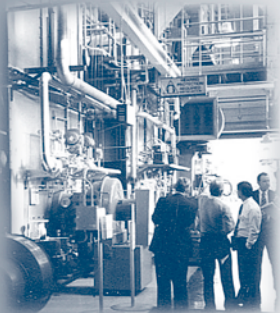
The slowdown on boiler blowdown. See page 5.
