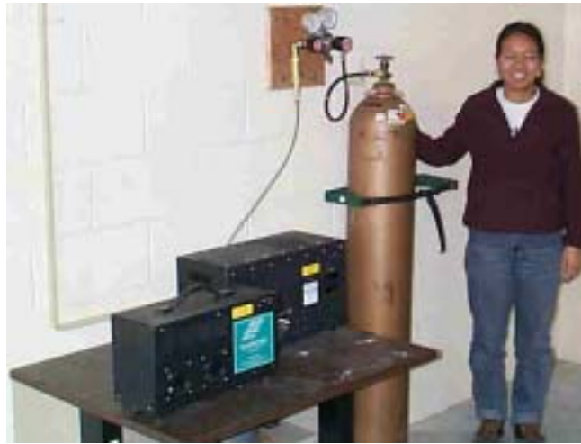
Figure 6. Installed fuel cell
