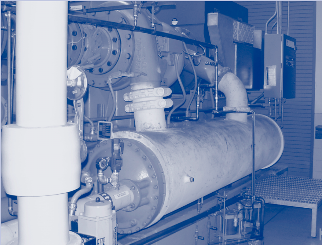
One of the 1,250-hp compressors in the Mehoopany mill
