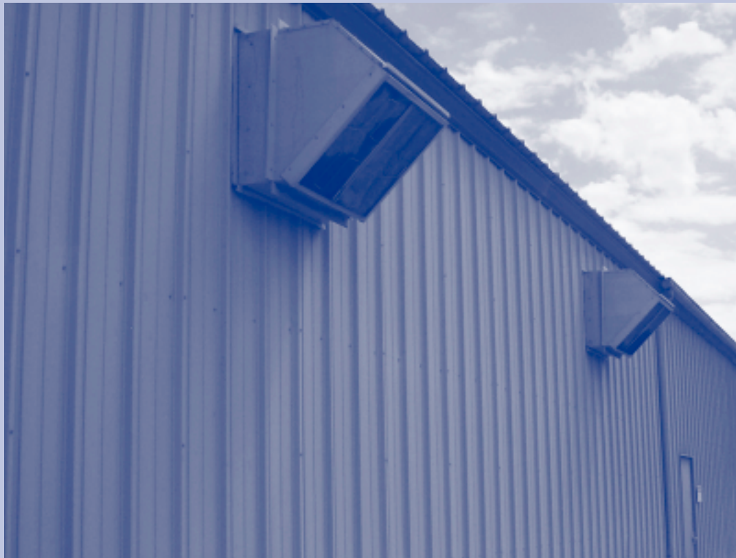
Ventilation Filters on Compressor Room Filter Wall
