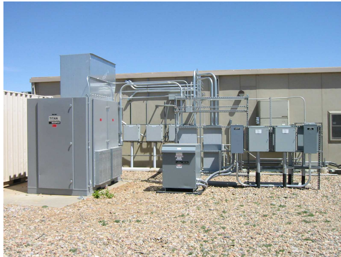
Figure 7. 165-kW Titan load bank (on left)
