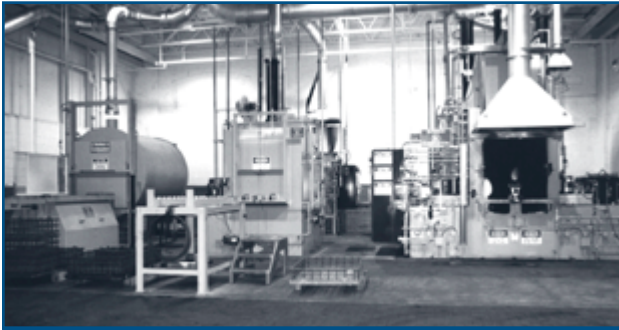
Quench Furnace Line for Heat Treating
