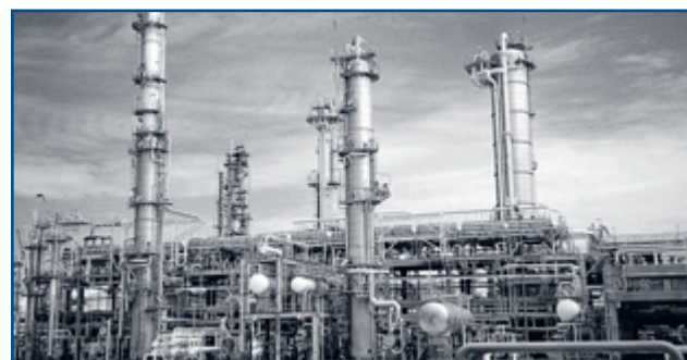
Fluid Heating in a Petroleum Process Heater
