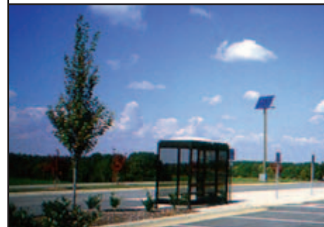
These stand-alone photovoltaic systems powered parking lights are an energy-saving alternative to traditional electric-powered lights in areas with adequate solar resources.
