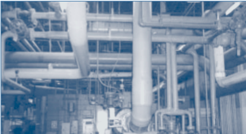
Inlet line to air compressor
