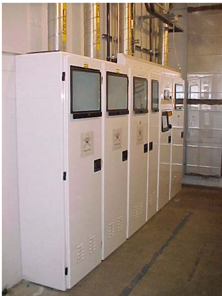
Figure 15. Automated cabinets for larger cylinders.
