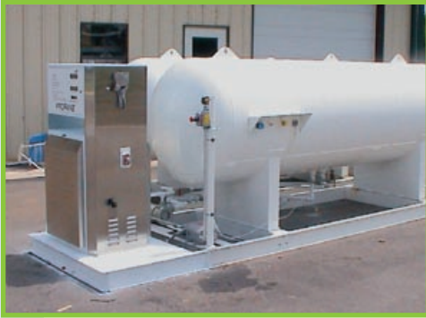
Propane is stored in above-ground tanks.
