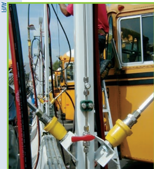
Type 2 nozzles are usually found in onsite fleet fueling facilities.
