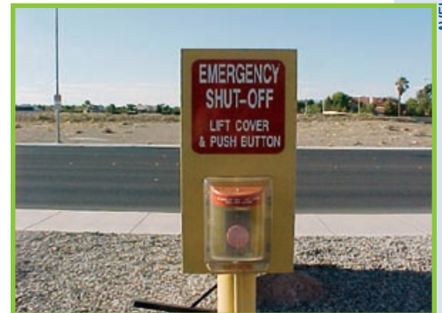
The emergency shutdown device stops the flow of natural gas to the pump. Drivers should take notice of the location of the emergency shutdown device at the stations they frequent.
