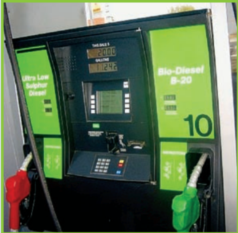
Fuel pumps require no modification to dispense biodiesel. Here, B20 and conventional diesel are dispensed side by side.
