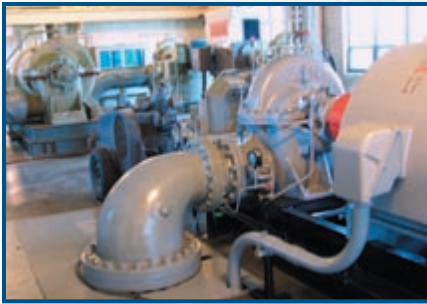
Lake Station high-lift pumps
