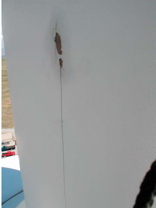
Figure 8. CART blade crack. The total crack length is approximately 59 cm.
