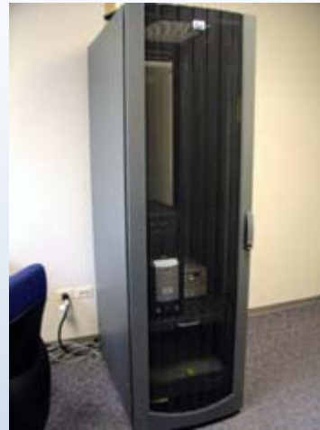
Server, workstation, tape backup and UPS
