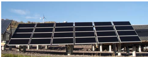
Fig. 1. Typical OTF rack mounted PV system.
