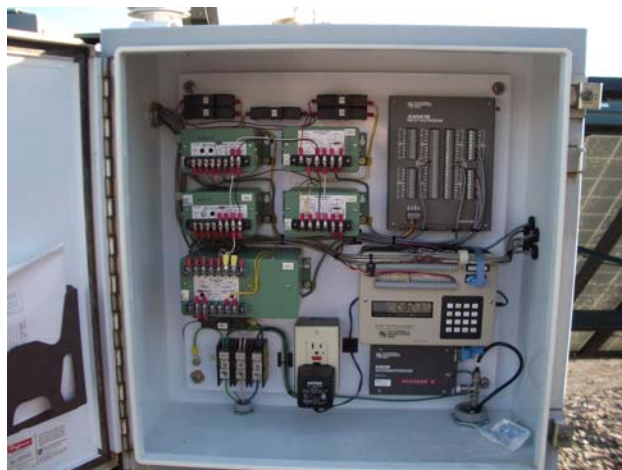
Fig. 2. Typical DAS using Campbell Scientific data logger.
