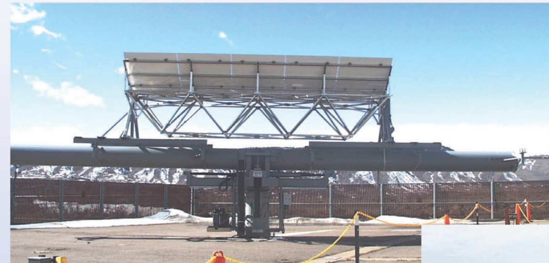
Tracker with Solargenix trough aboard
