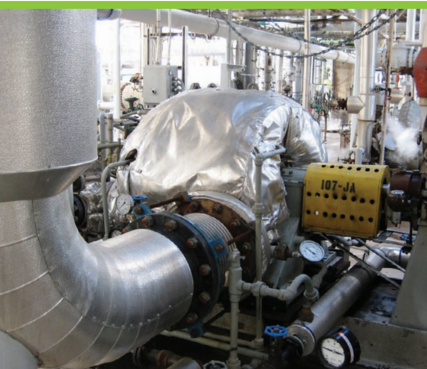
One of the new condensing turbines in ammonia plant #2; these new turbines are reducing energy use by 228,000 MMBtu annually.
