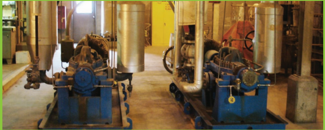
The J.R. Simplot Don plant in Pocatello, Idaho, repaired boiler feed water pumps such as the one pictured above, and revised boiler operating practices to reduce steam venting by 17 million pounds annually.
