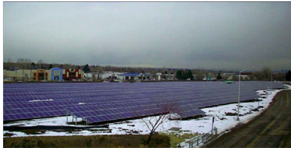
GSA Denver Federal Center (1.19 MWdc)
